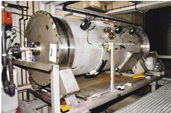
Technical size made of duplex steel with 3 m 3 /h flow since 2003 at the dolphinarium of Duisburg, Germany, with 3,000 m 3 volume
