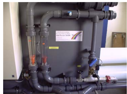
control panel with flow meters and valves
