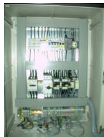
electric box with microprocessor control RO-matic
